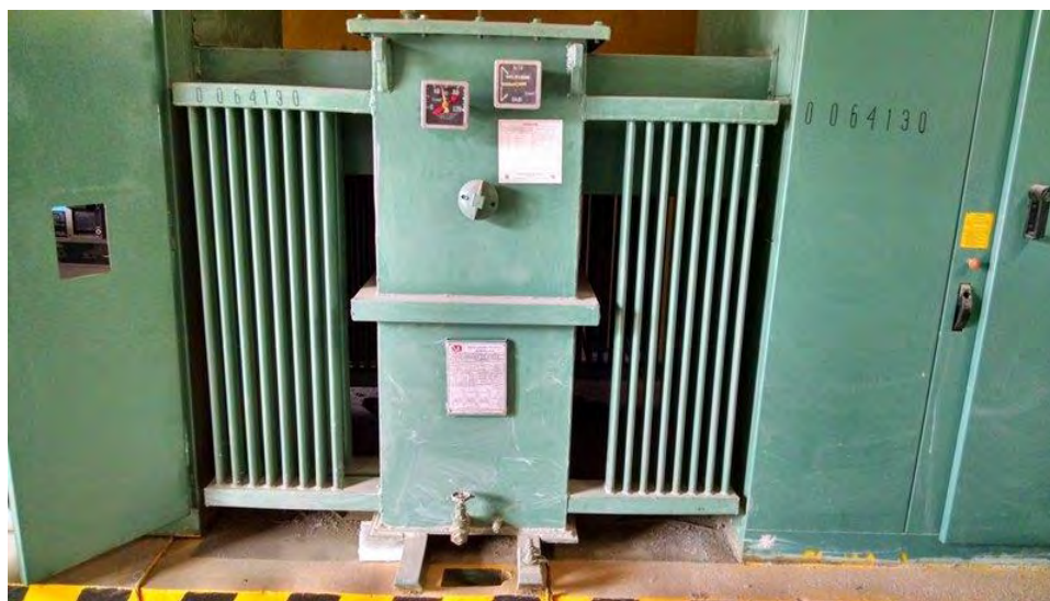
Figura 38 – Transformador principal del Hospital General ( Góngora, 2014 ).
