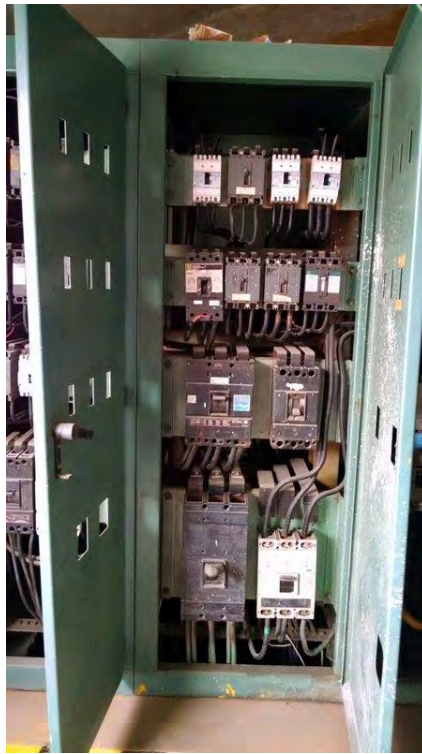
Figura 43 – Tablero principal (Góngora, 2014).
